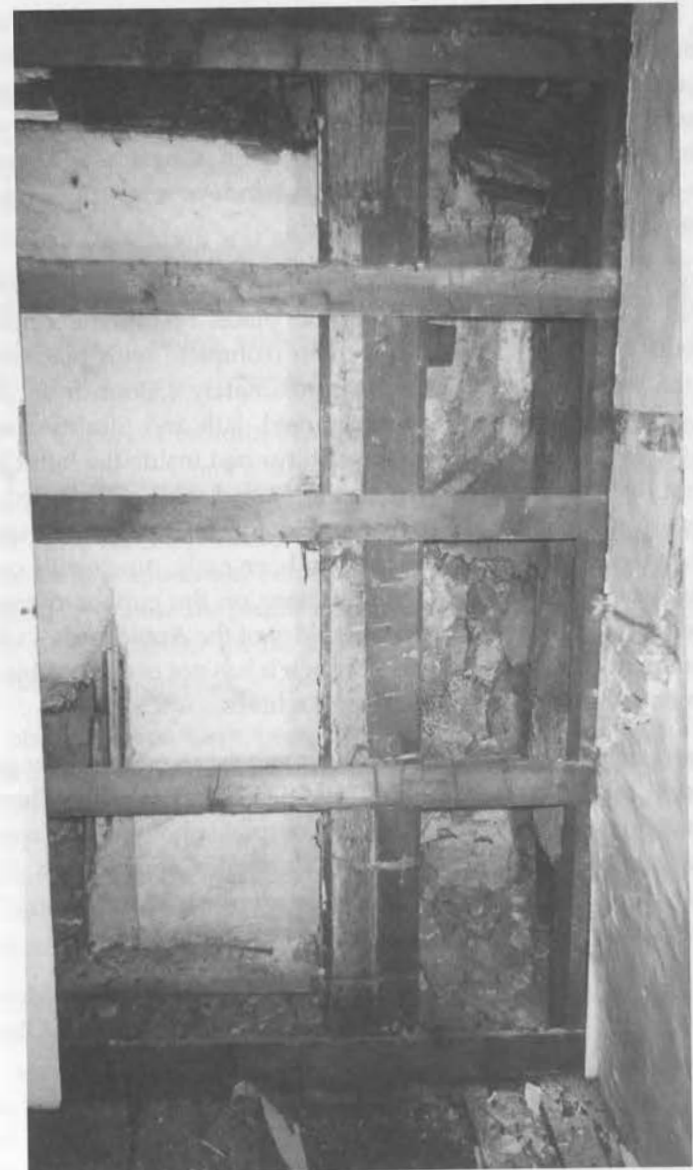
The void discovered in Second Court
